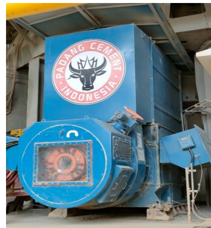
Gbr 5. Motor 6R1M03M1 HT WEG mill drive 6.3 kV 8700 kW
